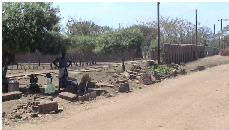
Figure 2: Shows a damaged walls fence of Kapalakonje Primary school in Nsanje District.
